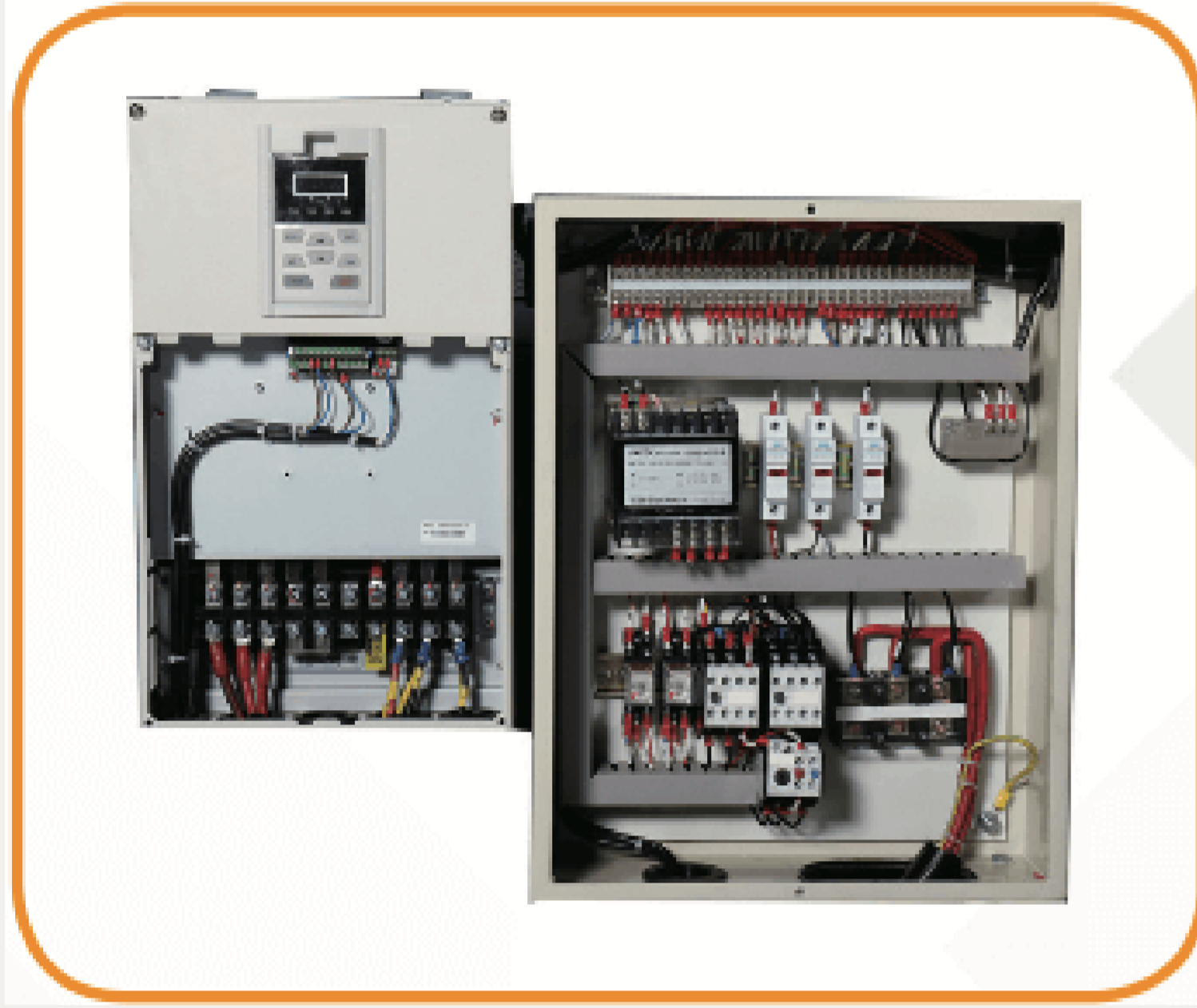
Inverter&Electric Inverter/PLC: Inovance
